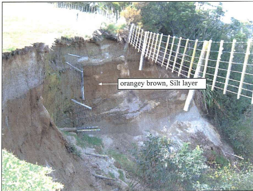
Fig. 2: Slip scarp along the south-western side of the subdivision displaying the distinct stratification of the volcanic soils.
