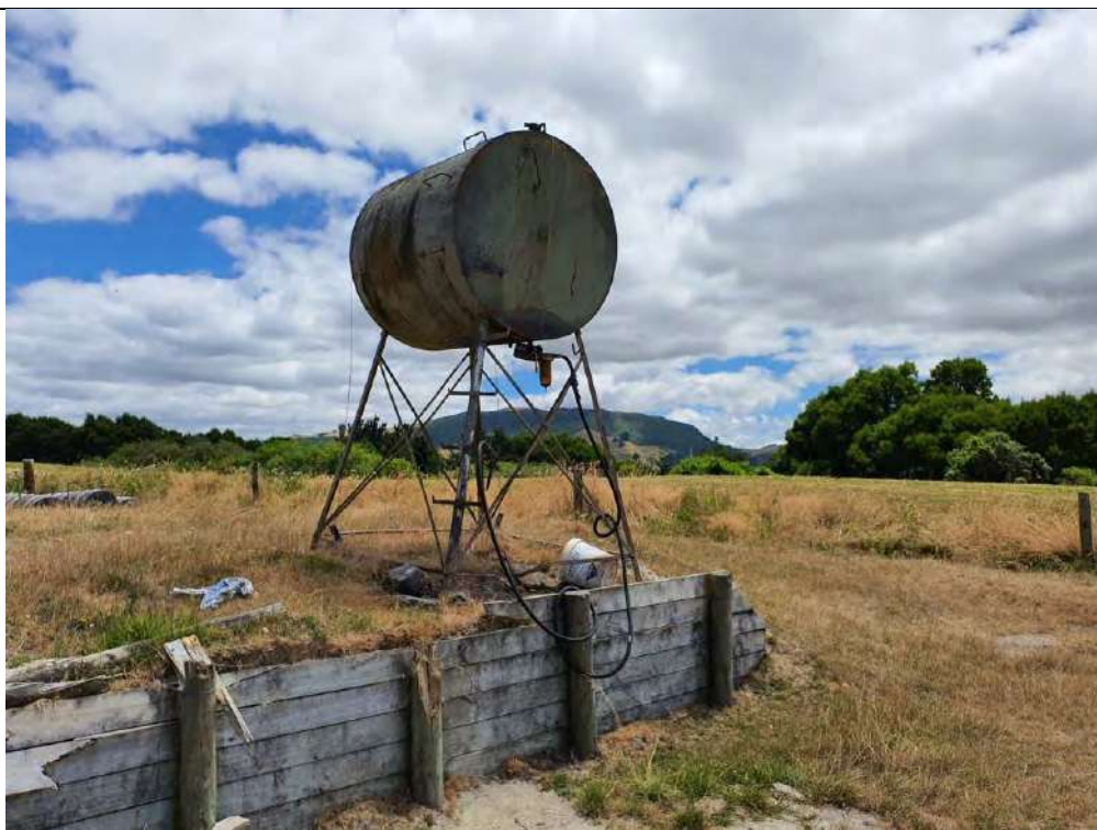
PLATE 3: Above Ground Fuel Tank
