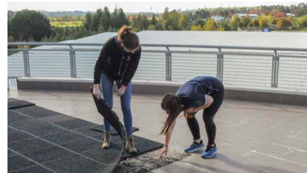
Above: Fitness and activities supervisor Doireann Meade and fitness instructor Kaitlyn Maxwell examine the tile damage at AC Baths
