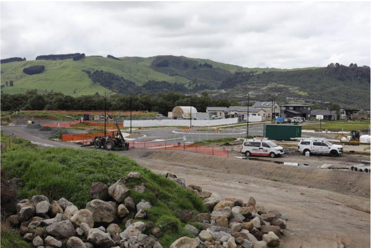
Figure 2: East from the constructed Okaia Drive roundabout. Locheagle Rise visible in the background.
