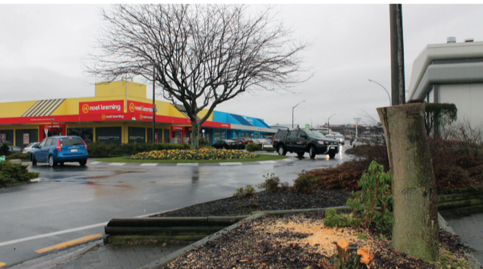
Above: Work at the intersection of Ruapehu and Tamamutu streets this week involved cutting down large trees obstructing views.
