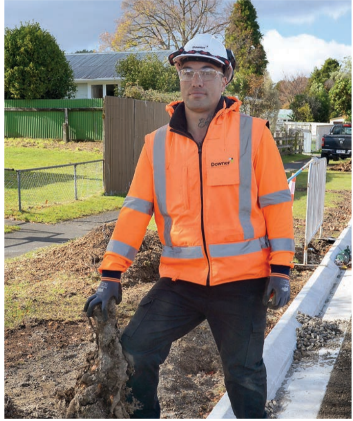
Out with the old and in with the new – Shaun Barnes with the damaged channelling in Turangi.
