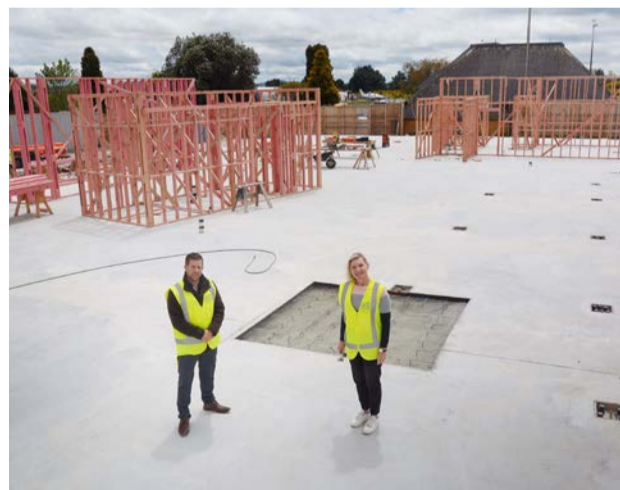
From left: Taupō Airport general manager Rhys Frearson and operations manager Kim Gard on the foundation of the new terminal building.
