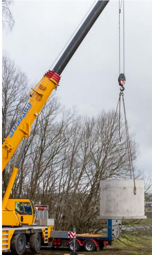
The components for Taupō's newest downstream defender were lifted into place on Tuesday morning.
